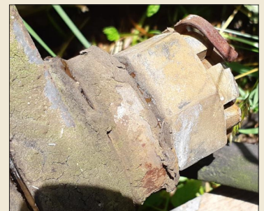
Fig. 5. Material Damage by Corrosion
